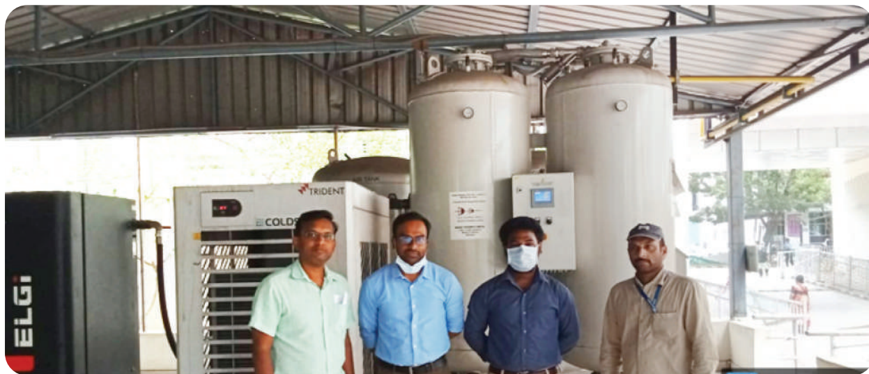
BDL installed oxygen generation plant at ESI medical college and hospital at Sanathnagar in Hyderabad
